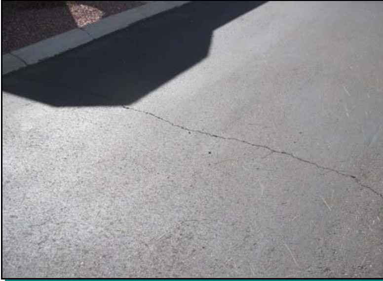
Transverse crack at Brookhaven Lane
