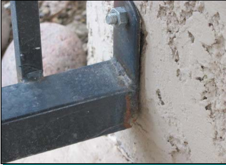
Rust at fence fastener
