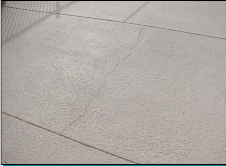
Concrete deck crack, note recent coating application
