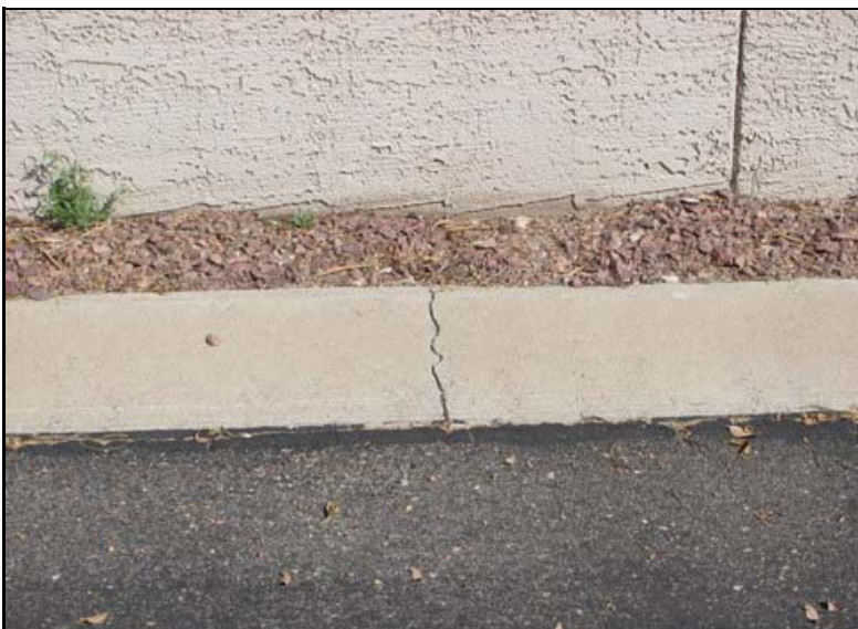
Concrete gutter crack at Cave Creek Drive
