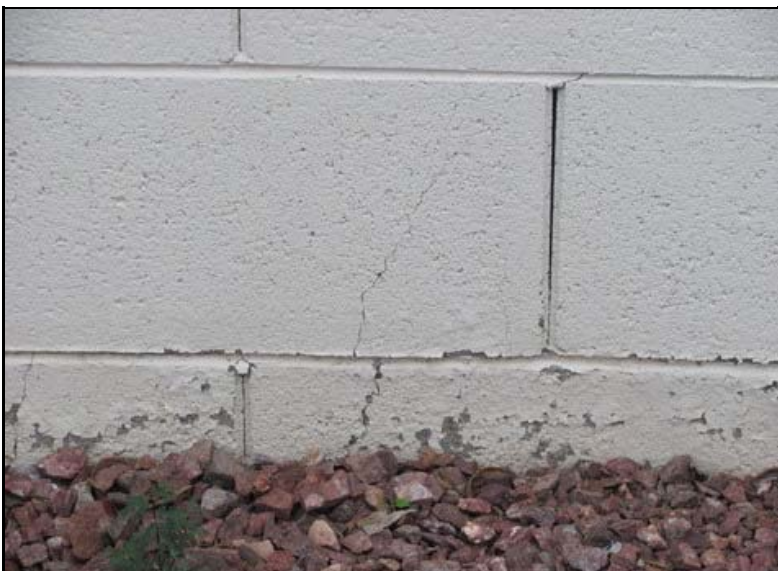
Hairline crack and paint finish deterioration at concrete blocks
