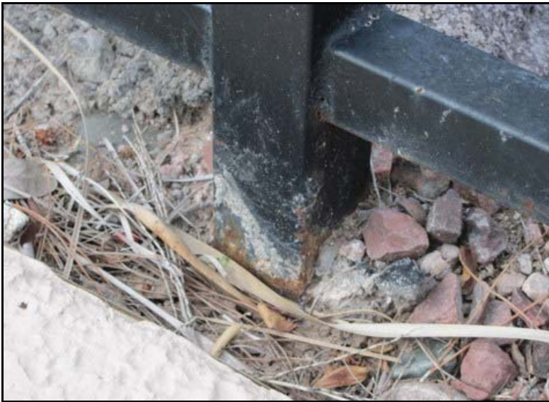
Rust at base of metal fence post
