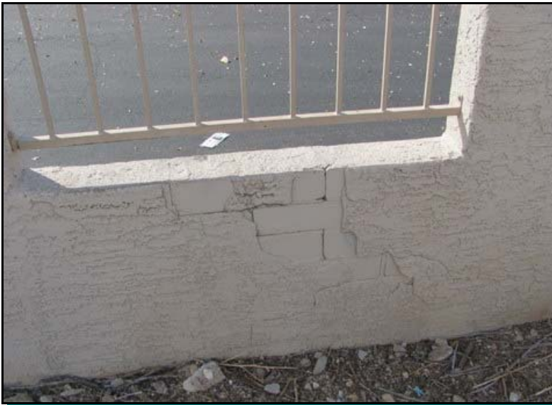
Step cracks and stucco deterioration
