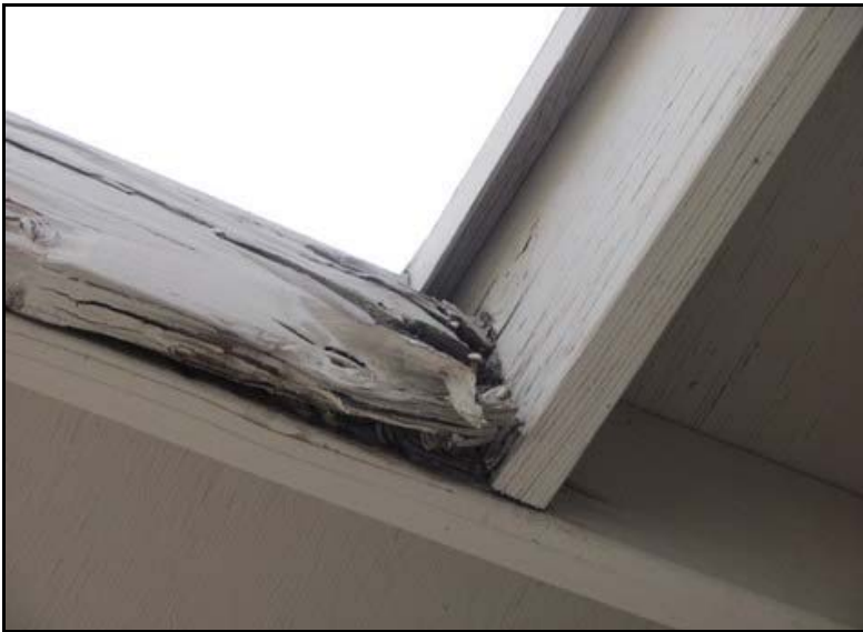
Deteriorated wood frame member at Ramada
