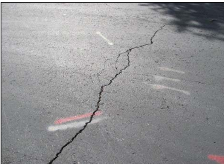
Transverse crack at East Dianthus Place
