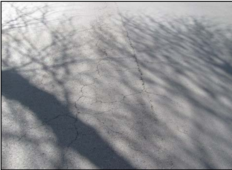
Fatigue cracks at East Dianthus Place
