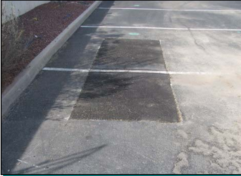
Previous patching at Bull Rush Lane
