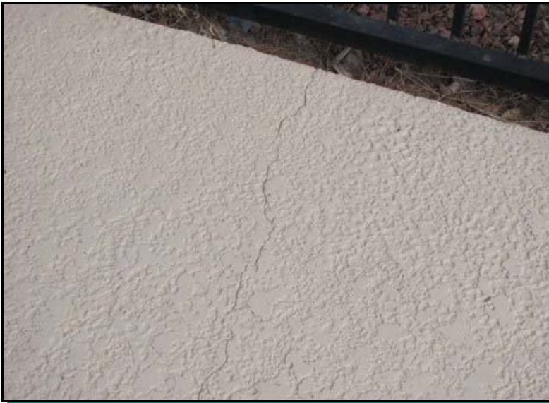
Hairline deck crack
