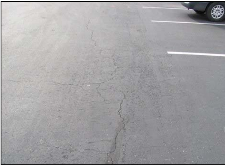
Fatigue cracks at Catalina Avenue
