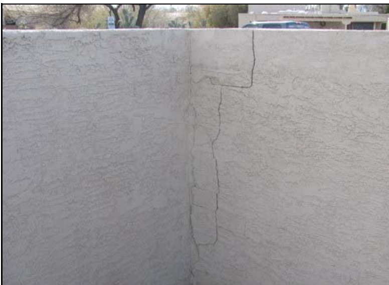
Cracks in perimeter wall corner
